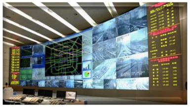
Emergency Command Center (72 Screens)
