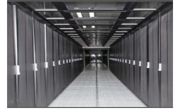
Data Center( 48 Racks)
